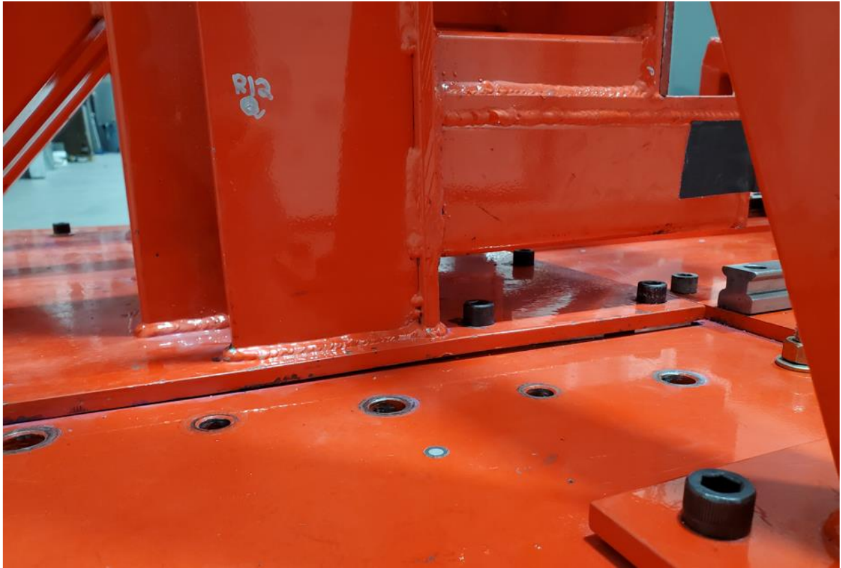
Figure 4. Detail of Calspan Base Plate Showing Gap; Calspan Added Shims at the Right Corner to Compensate for the Bending.
