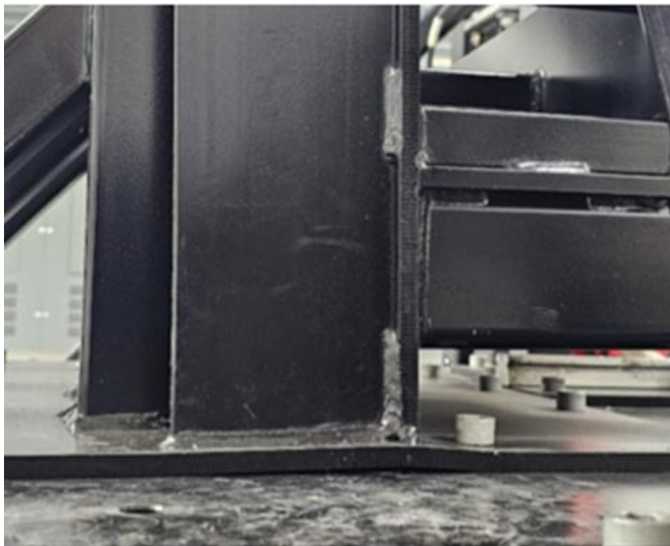
Figure 5. Detail of MGA-Virginia Base Plate Showing Gap.
