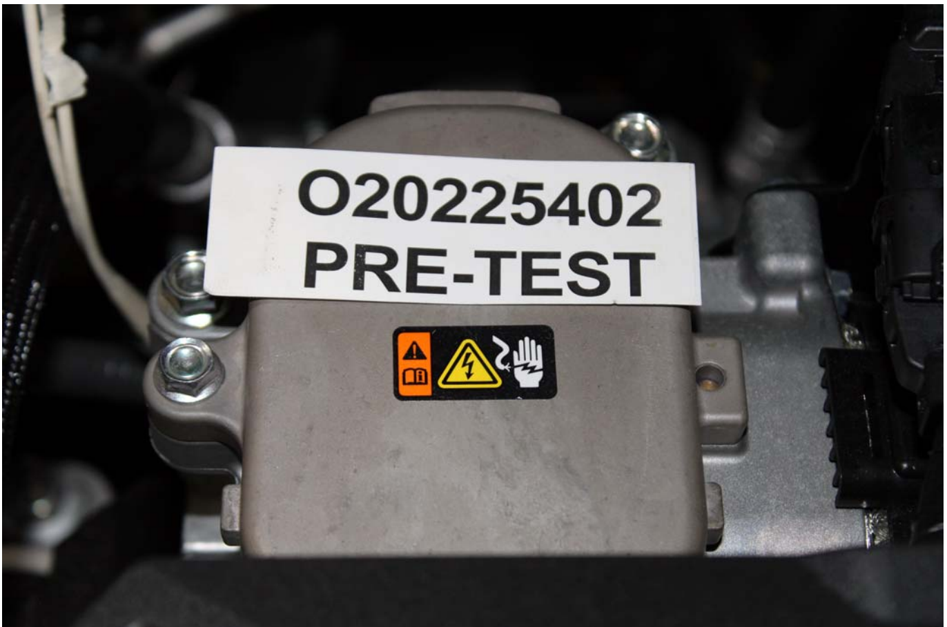
Photo No. 305-02 - Power Inverter Warning Label
