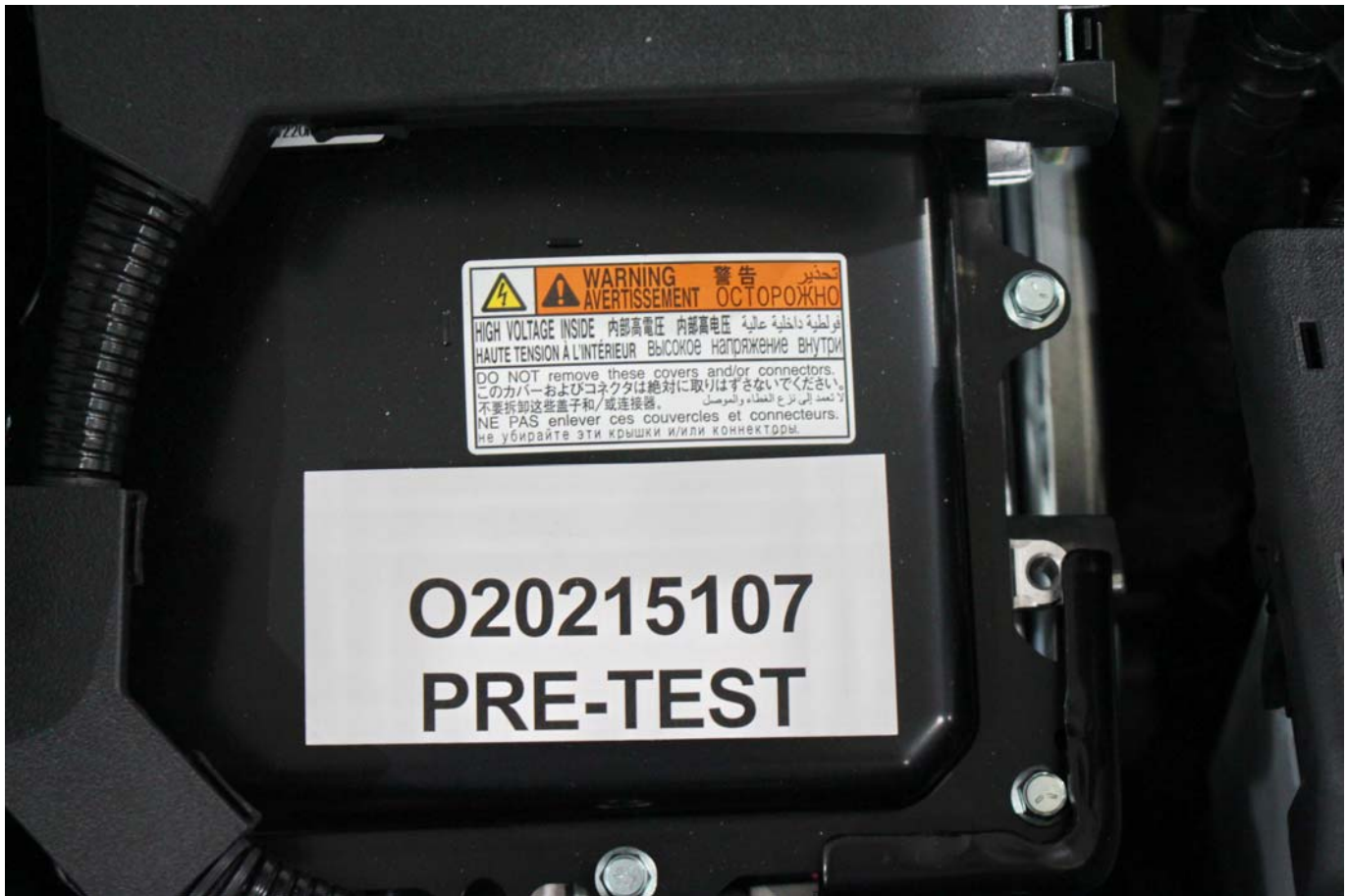
Photo No. 305-02 - Power Inverter Warning Label
