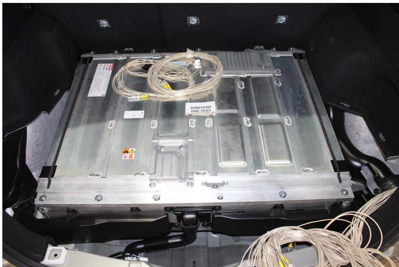
Photo No. 305-09 - Pre-Impact View of Propulsion Battery
