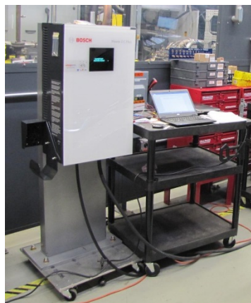
Figure 27: 24 kW IES (BOSCH) CCS Charge Station
